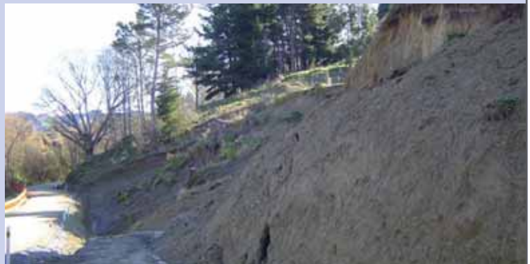
Work has begun on preventing further slips of the playing field at St Joseph's, Taihape
