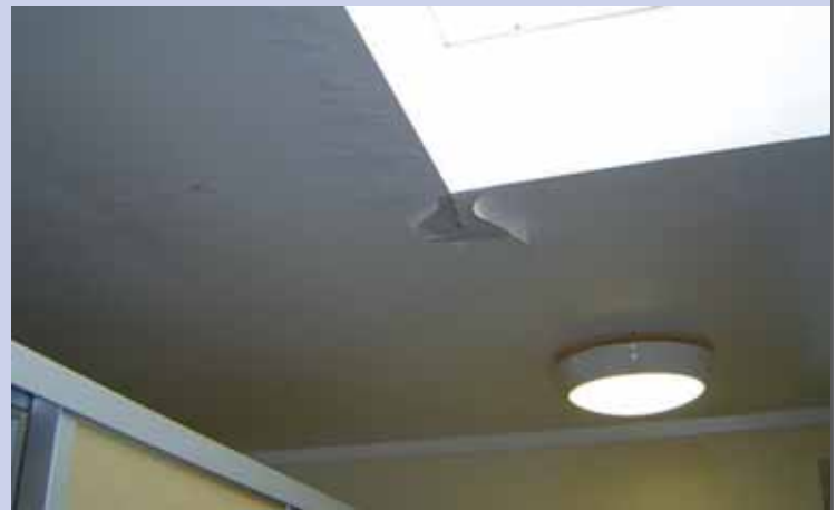
Damage caused by poor flashing around skylights
