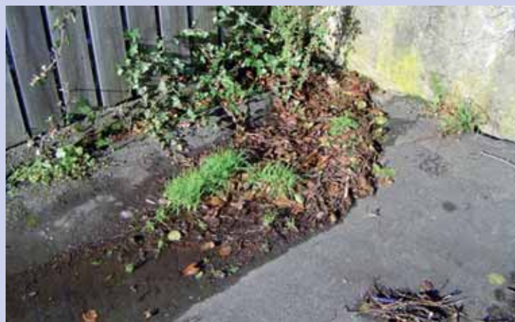
A grate drain is buried under here!
