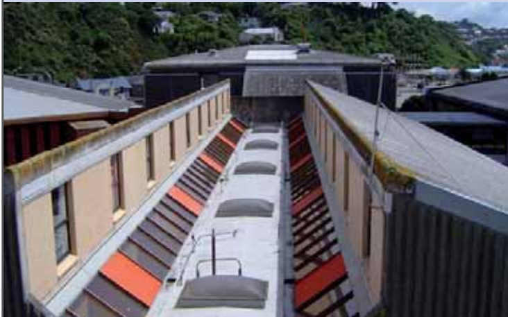
Extensive remedial work is planned for roofs at St Patrick's College, Kilbirnie
