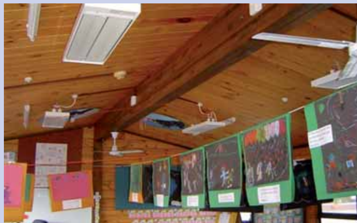
St Theresa's Plimmerton classroom overhead convection heating (and nice artwork!)
